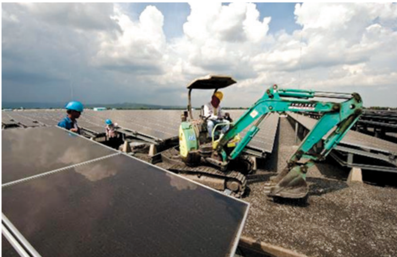
Figure 10: Solar power project in Thailand. The 73-megawatt Lopburi Solar Farm is one of the largest photovoltaic projects in the world. The Lopburi Solar Farm is integral to Thailand's efforts to generate energy from renewable sources. Credit: Asian Development Bank (CC BY-NC-ND 2.0)
