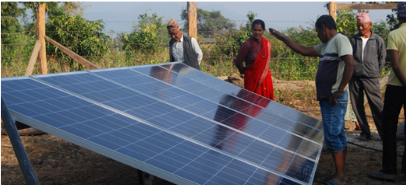
Figure 15: The installation of solar-powered irrigation system in Nepal to collect water from the river to a pond which will be used for irrigation during the dry seasons. Photo Credit: Shobha Manandhar
